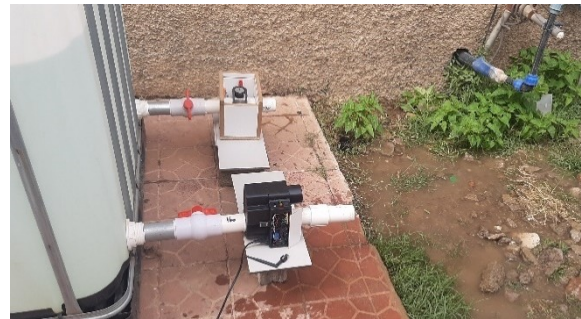
Figure 12. Real test of closing solenoid valve
